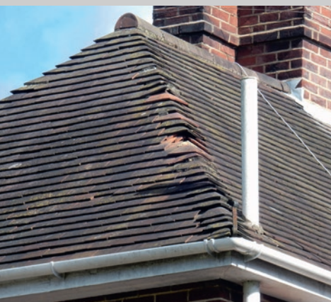
Slipped and loose roof tiles
