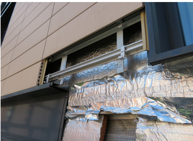
Figure 10: Typical build-up of terracotta rainscreen cladding (note missing cavity barriers around window openings)
